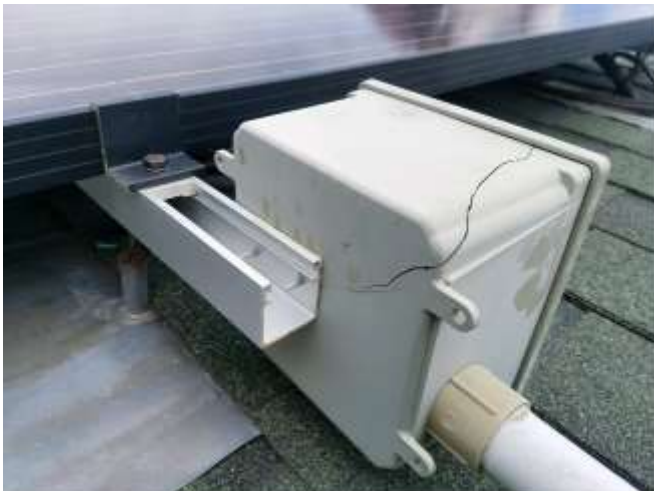
Figure 1 damaged junction box found during visual inspection. This was filled with water and caused the system to trip off line
