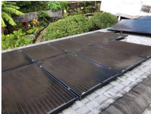
Figure 1 panels that were not cleaned and have major mold build up – they are not getting any sunlight
