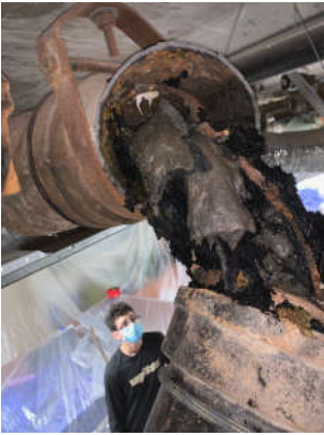
Clog in an opened DWV pipe
